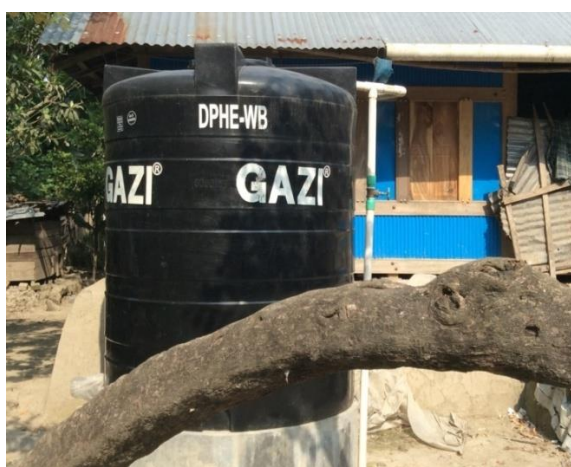
Figure 3.5: Photograph of Rain water harvester in Nishanbaria union
