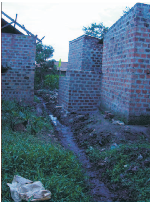
Figure 4. Material from ordinary pit latrines or dry latrines should never be excavated and drained away in drain gutters. Human exposure to faecal contamination in storm-water drains is a major risk for transmission of enteric and parasitic diseases.
