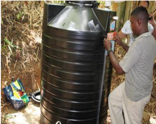
The worker is seen here connecting a water level indicator to the RWH system.
