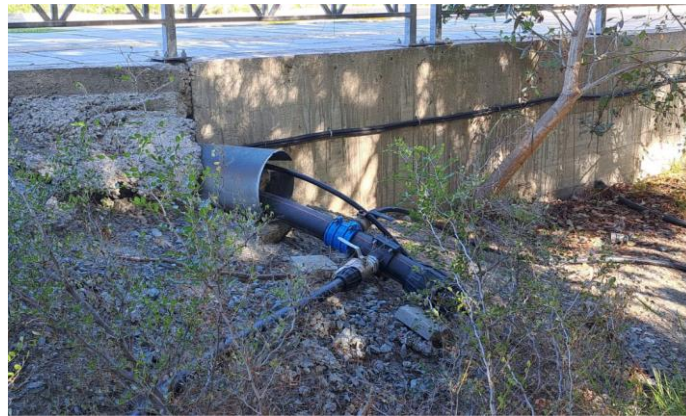
Picture 1. Treated wastewater inlet in the park.
