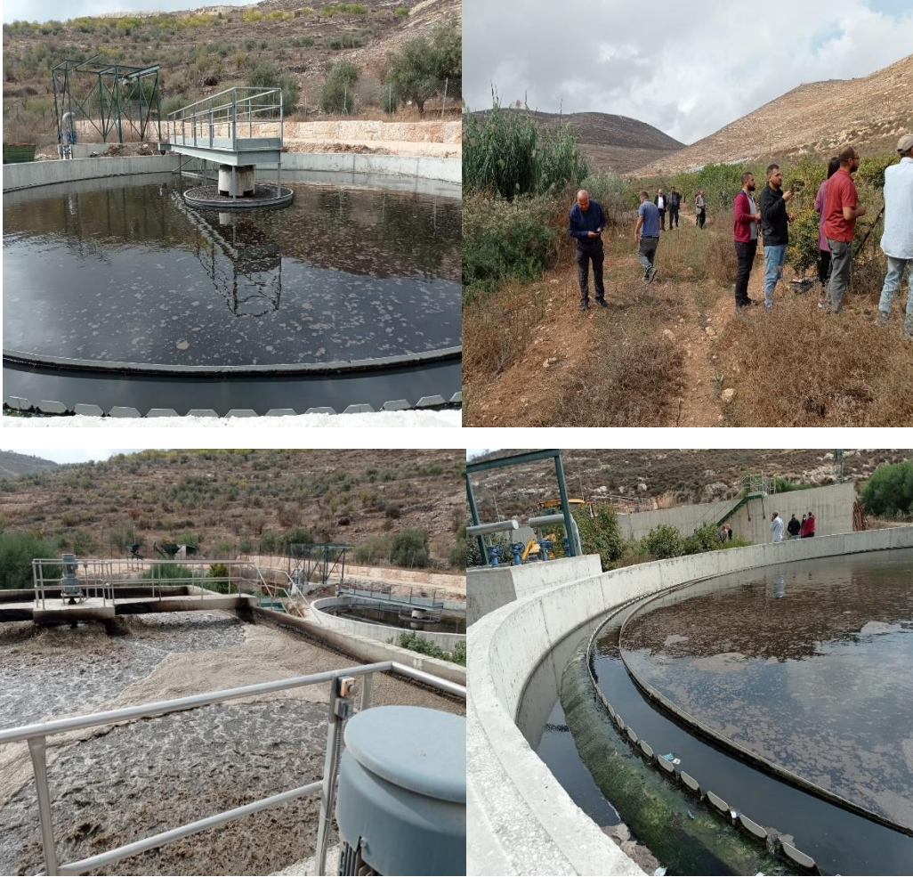
Al-Arroub Plant wastewater treatment at Sier, Hebron / Palestine
