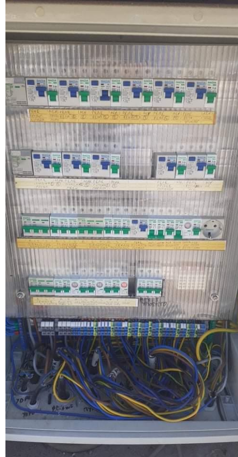
Figure 5. The internal components of the electrical board.
