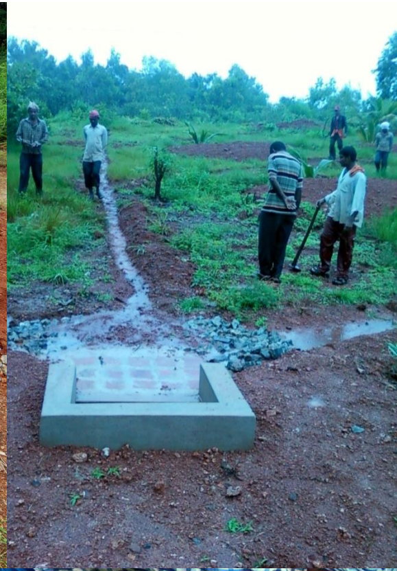
Storm water Filter
