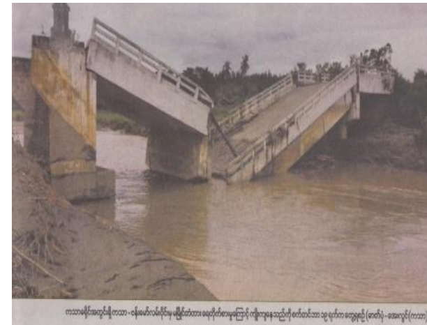
Damage of Bridge in Sagaing Region
