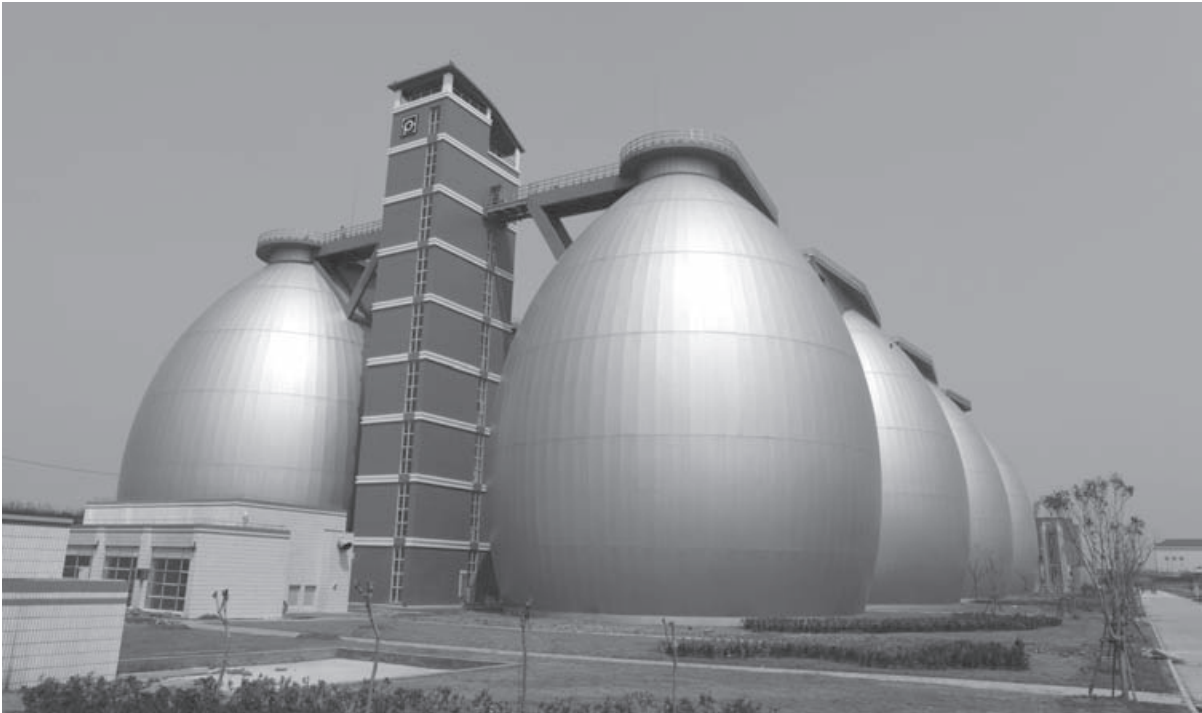
Resources and energy from sludge should be recovered where this is economic. Above, sludge digesters with biogas recovery in Zhujiajiao, Shanghai.
