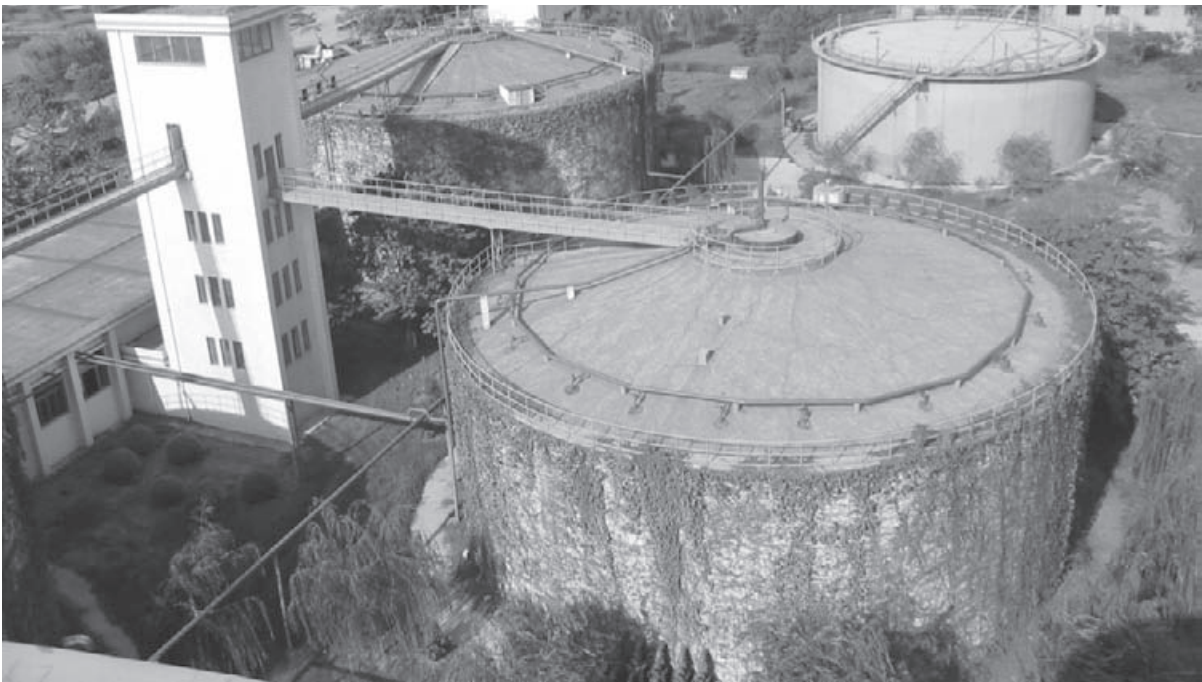
Anaerobic digestion of sludge with biogas generation and utilization is commonly adopted to stabilize sludge. Above, sludge digester at the Sibao wastewater treatment plant in Hangzhou, Zhejiang Province.
